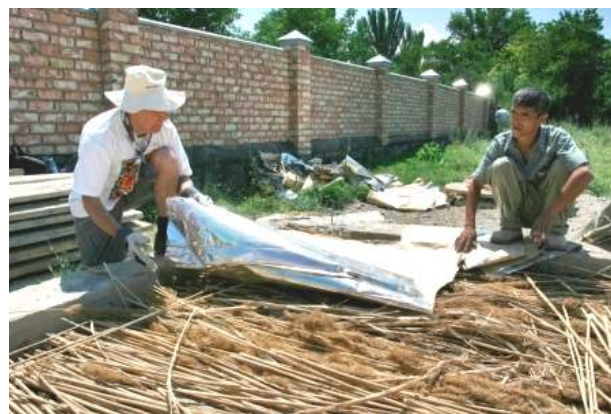
The volunteers cover folic paper and pour more cement on the floor.
